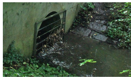
Figure 2: The end of the cylindrical pipe is hidden by a grid
