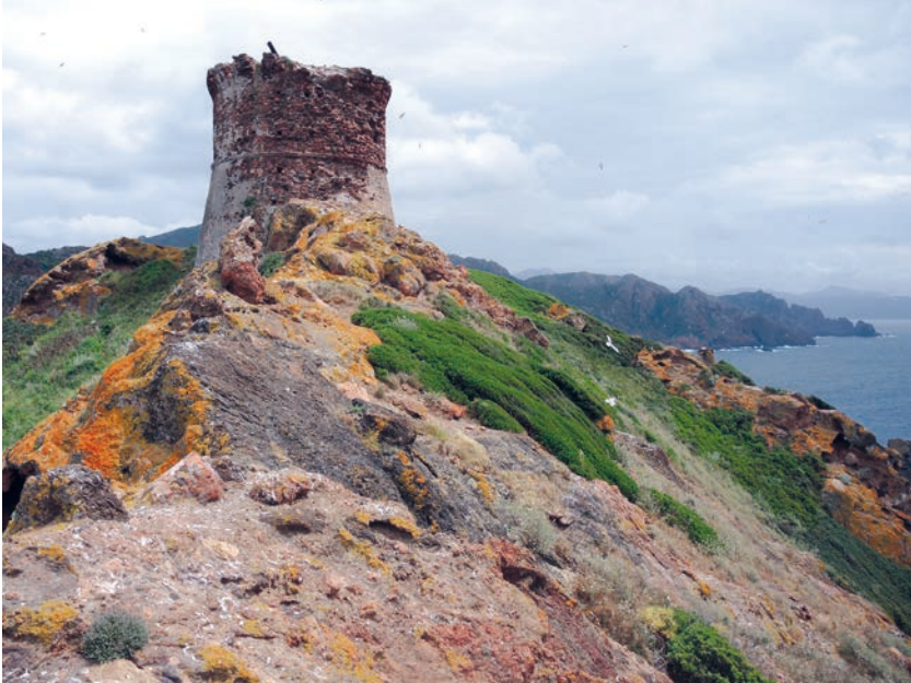
Figure 8. The Genoese tower on Gargalu Island, in the core of the Scàndula Nature Reserve. Its construction in about 4 months in 1610, on a steep island, without water, without food resources, without wood, without limestone for lime, was a technical feat. In the near background, Gattaghja Bay and Punta Muchilina. In the far background, the southern shore of the Gulf of Portu, with the Calanche di Piana. Photo © Frédéric Médail.
